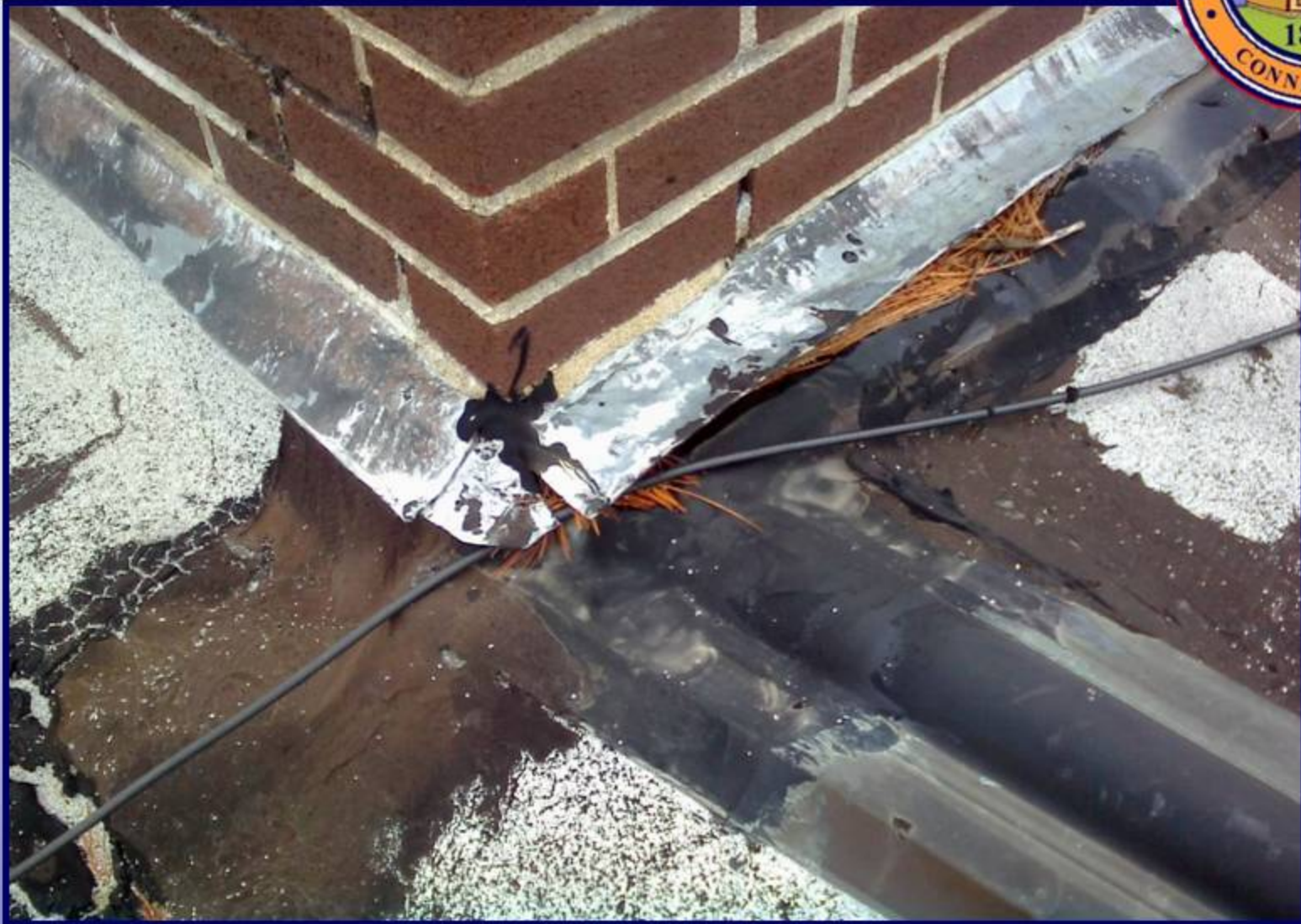
Deteriorated flashings and masonry
