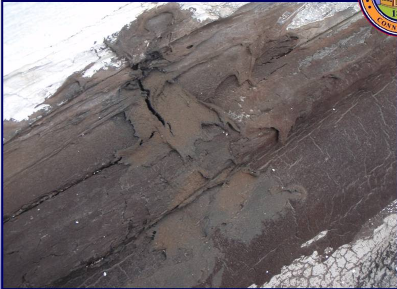
Deteriorated roofing; patching to prevent leaks
