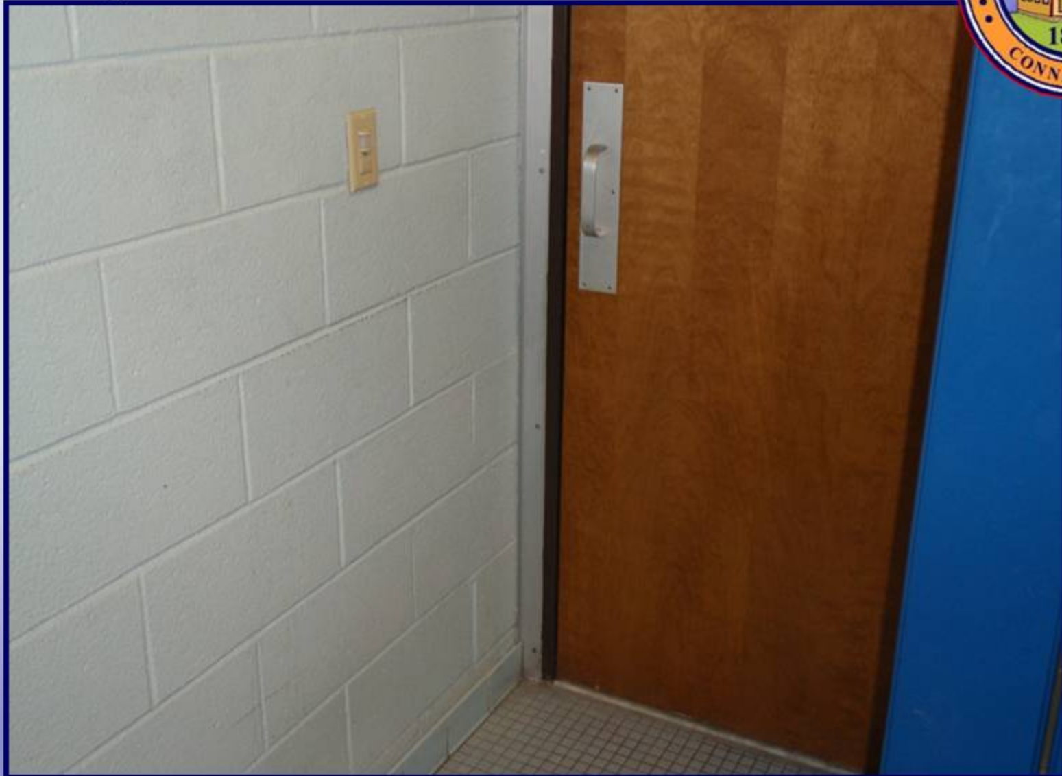
Latch-side clearance issue at multiple locations
