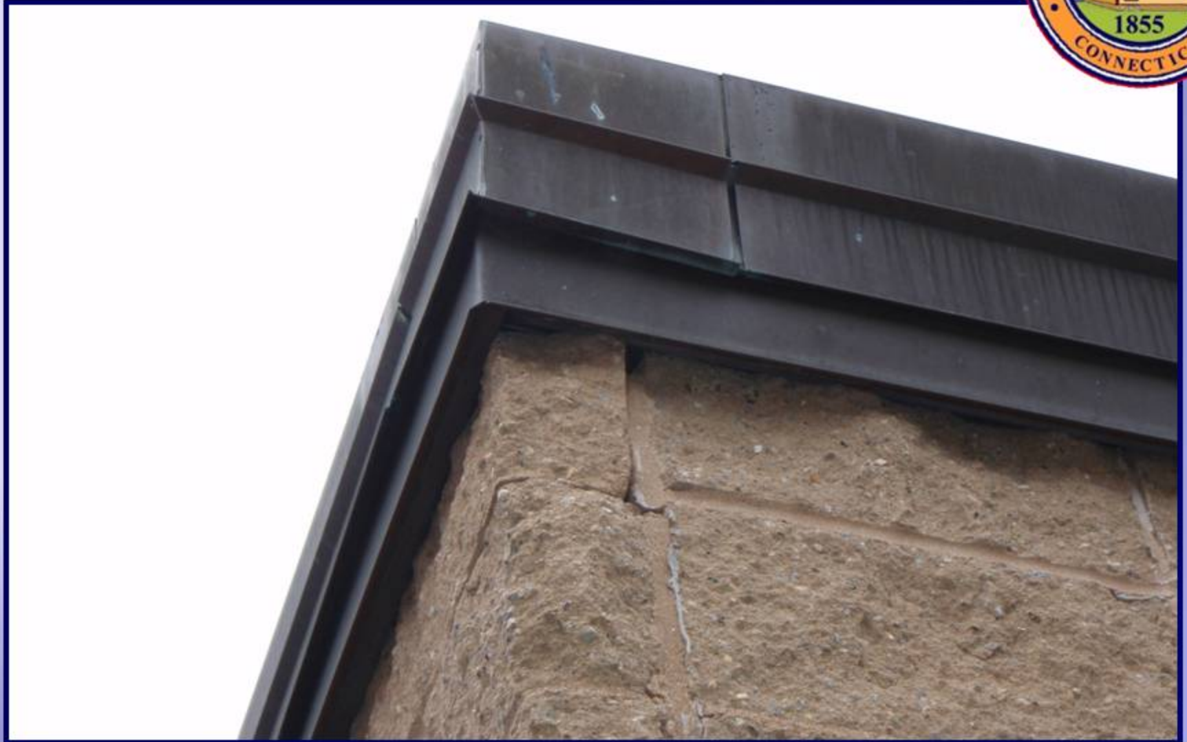
Deteriorated masonry at corners
