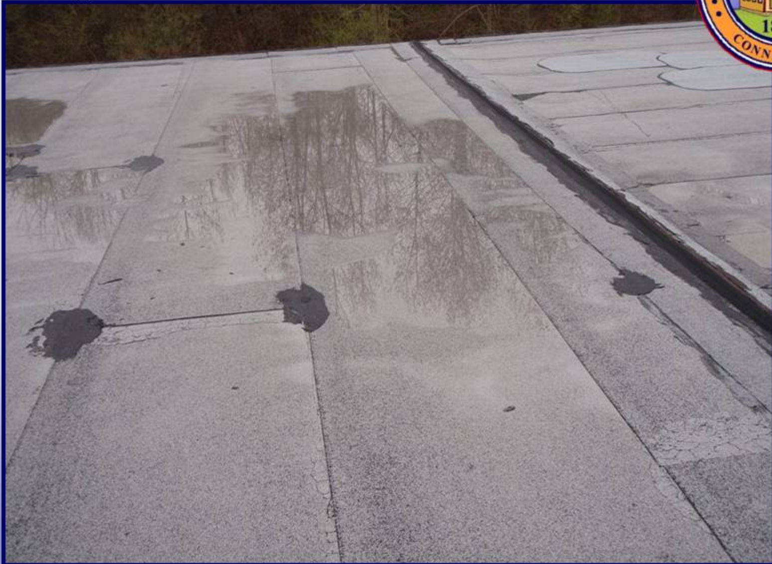
Ponding water on existing roof; poor slope to drains
