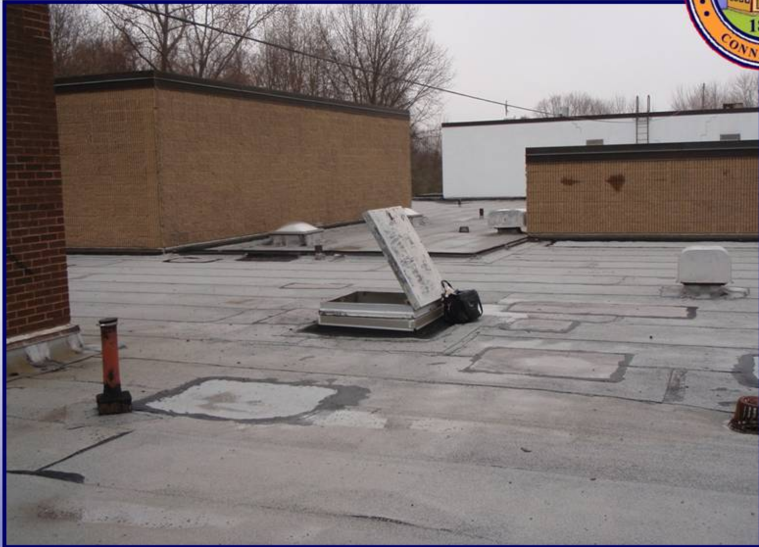
Existing roof; multiple patches; multiple leaks
