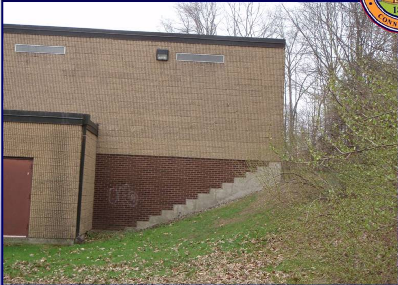
Grade causes surface water to drain towards rear of building
