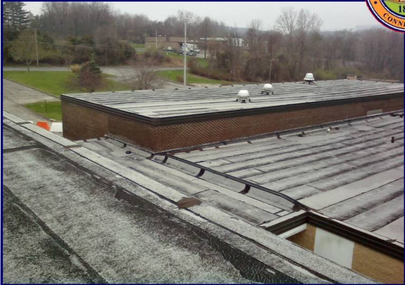
Roof has many leaks
