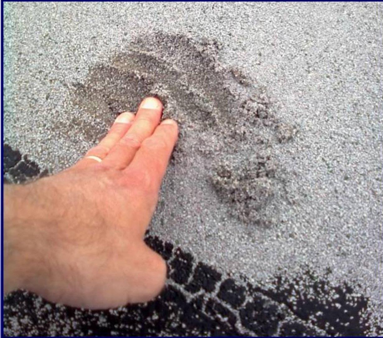
Granular material from deteriorated roofing
