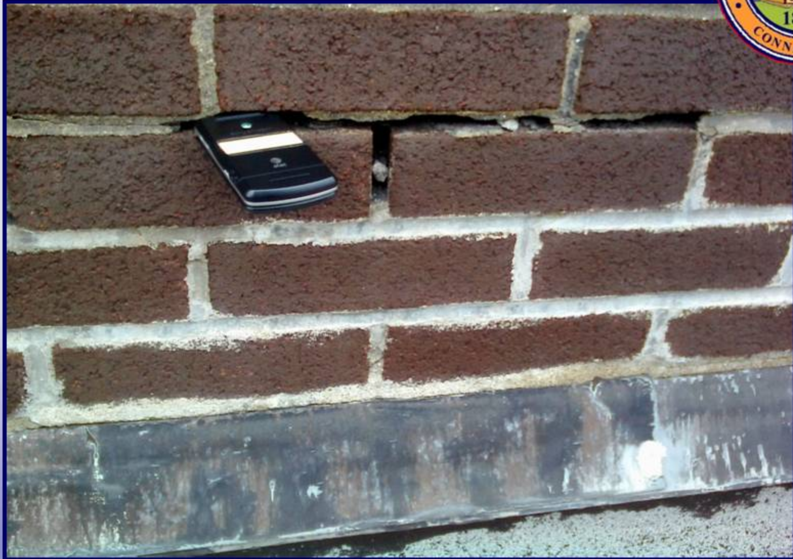
Small areas of deteriorated masonry joints
