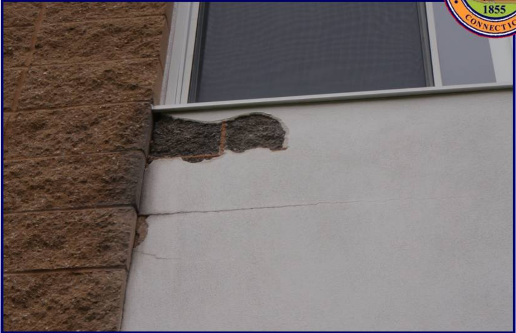
Deteriorated plaster stucco finish below windows
