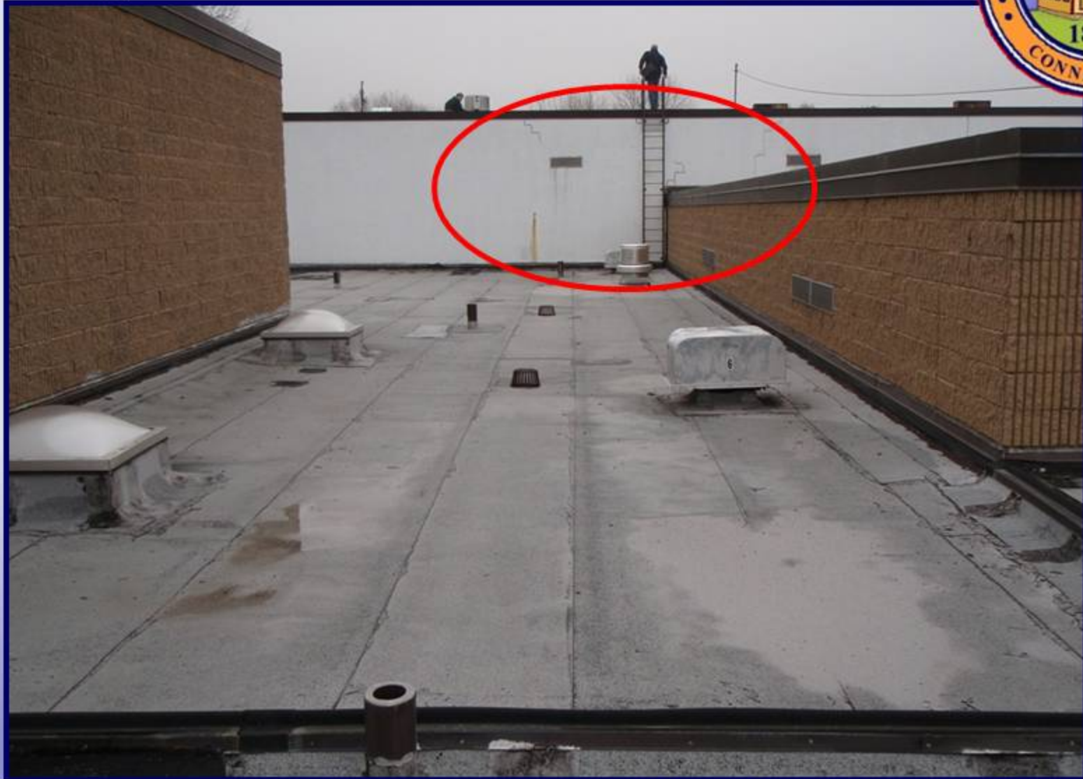
Area of step-cracks in masonry sidewall of Media Center
